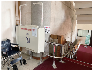
裝裝置無障礙升降平臺提升友善使用環境 Installation of barrier-free lifts to provide a more user-friendly environment.
